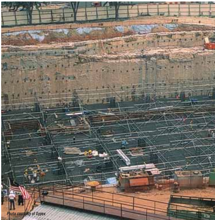
Excavation and diaphragm wall for Maybank Headquarters, in Kuala Lumpur, Malaysia. Architect: Hijjas Katsuri; courtesy Xypex.
