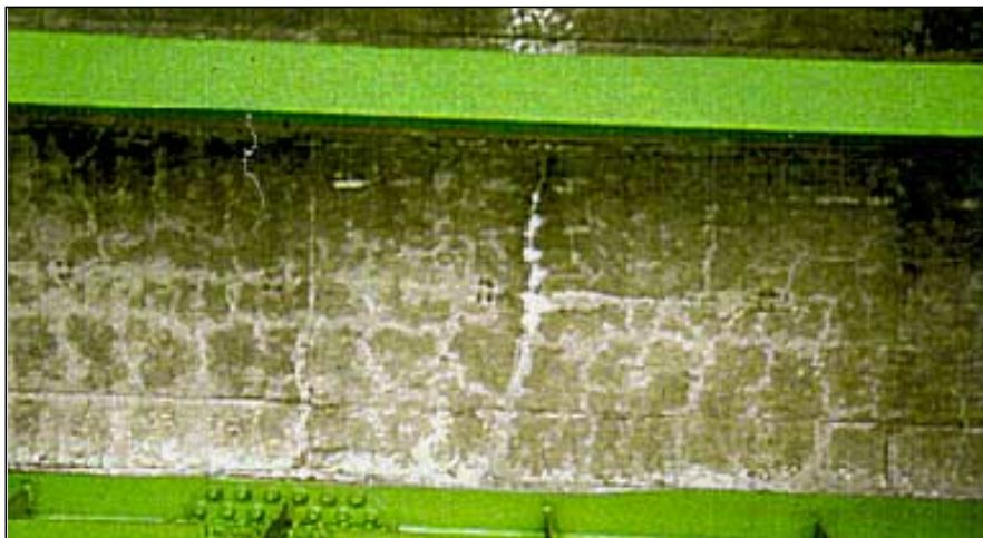
Photo 1: Evidence of cracking in concrete on underside of the deck slab
